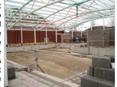
The mild winter has allowed for time to be made up on the construction of the North Herefordshire Pool caused by the delay in the steel reaching site.
